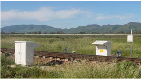
Figure 3: Photograph of ARTC's RailBAM® Installation at Nectar Brook
